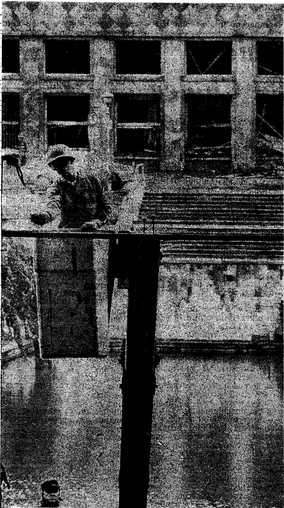
MORNING-AFTER CLEANING UP — An engineer soldier removes glass shards from window frames after the explosions which shattered many windows in the I. G. Farben Building the previous night. Spec. 5 Mike Pitschke made this photograph, showing the reflecting pool and wrecked facade of the Terrace Club.
